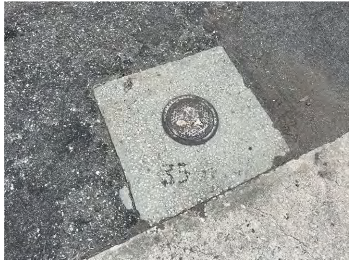
PHOTOGRAPH 6 View of one of the groundwater monitoring wells (MW-35) on the subject property.
